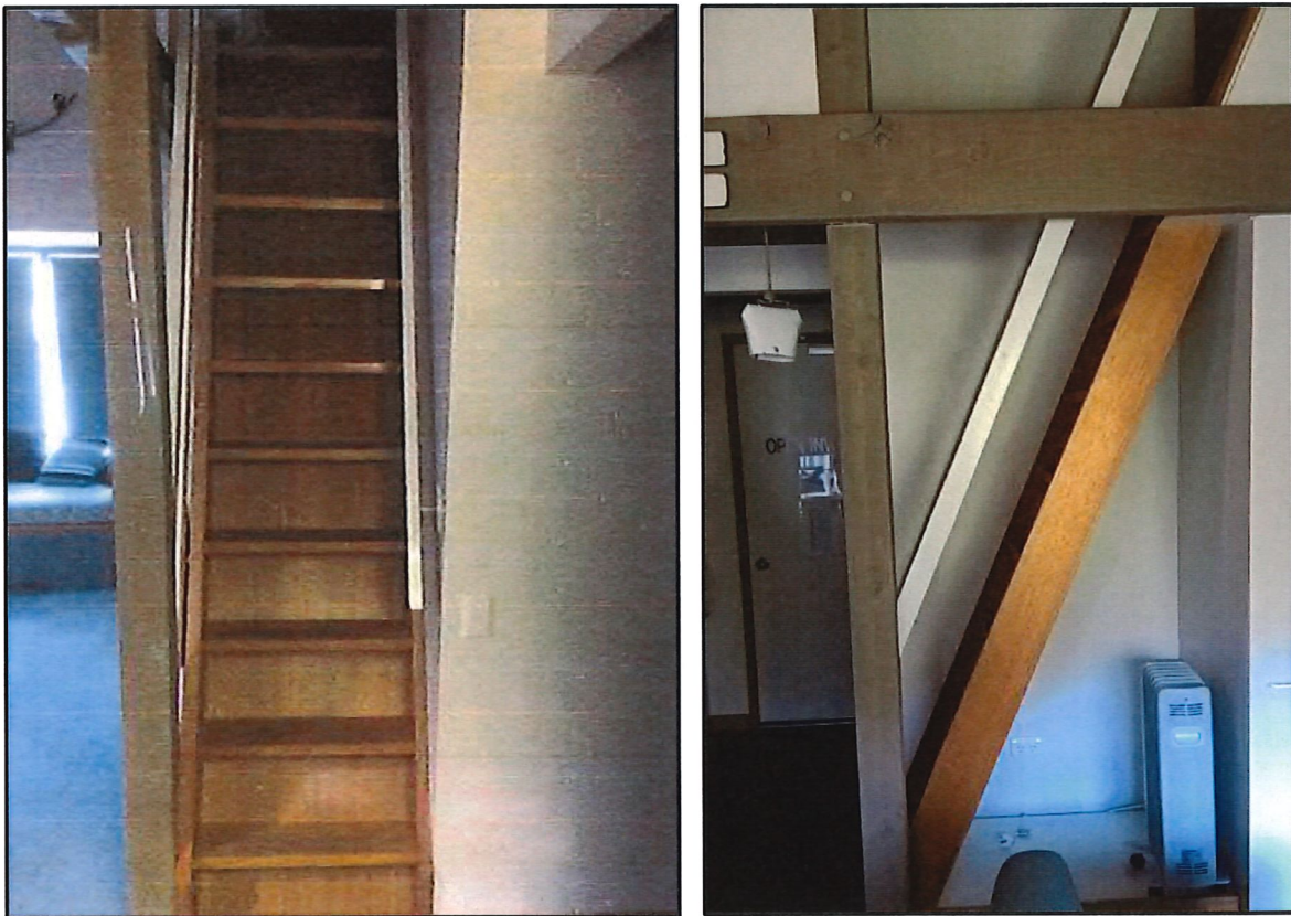
Figure 3: Existing ladder proposed to be replaced (Source: DPE inspection photo and applicant SEE)
